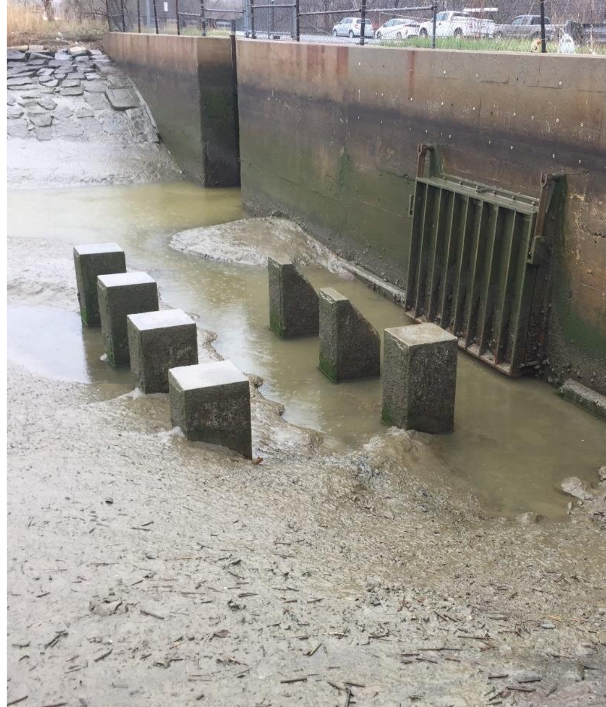
Outlet of Sales Creek to Belle Isle Inlet; Existing DCR Tide Gates
